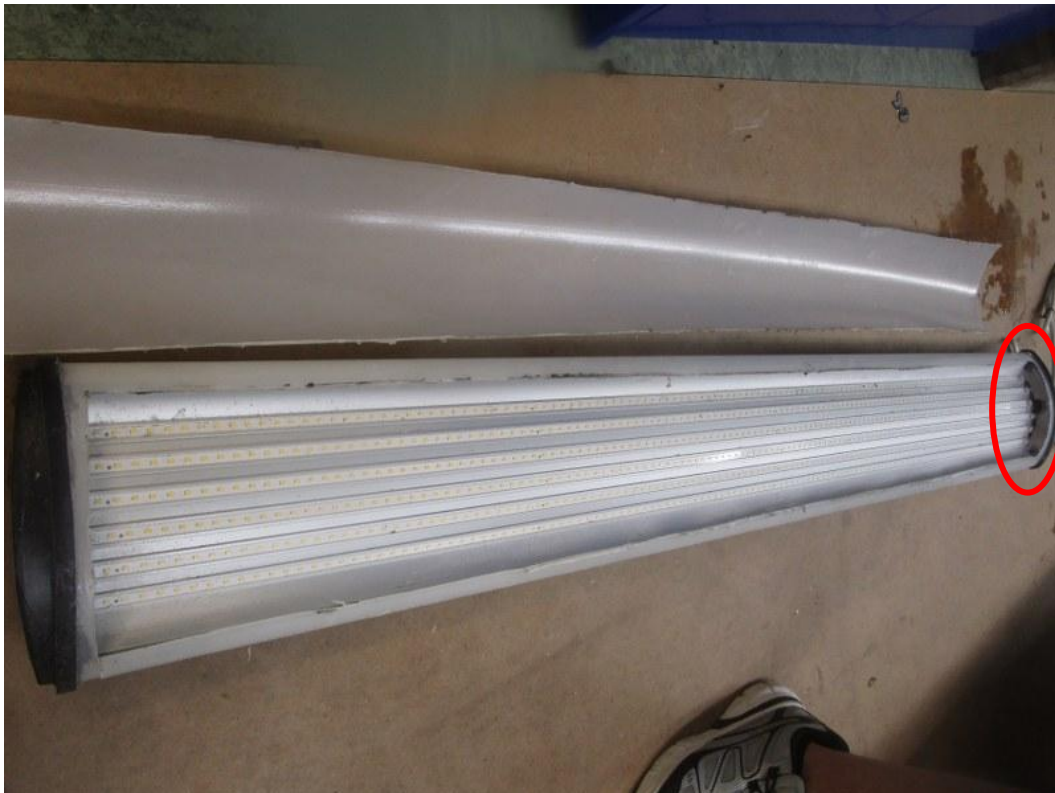
Photo 17 Visual inspection. Water observed behind the end cap. Not visible at photo.
